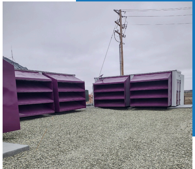
Bitcoin mining containers located at the Hardy substation.
